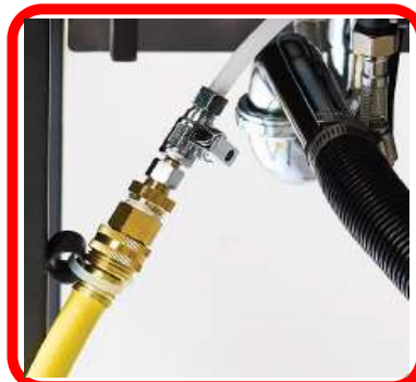
ALL PIPES & VALVES READY TO CONNECT
